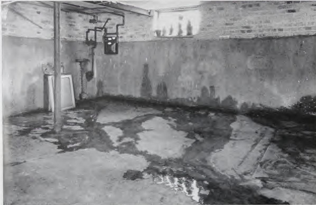
An actual photograph of a damp basement. The use of Medusa Waterproofed Gray Portland Cement would have prevented this condition.
